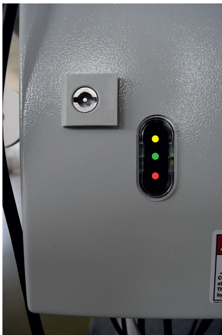
Fig. 1: LEDs on the control cabinet
